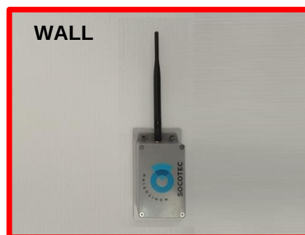
Fig.7 : bad installation (front view)
